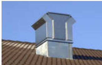
Mechanical smoke extraction
