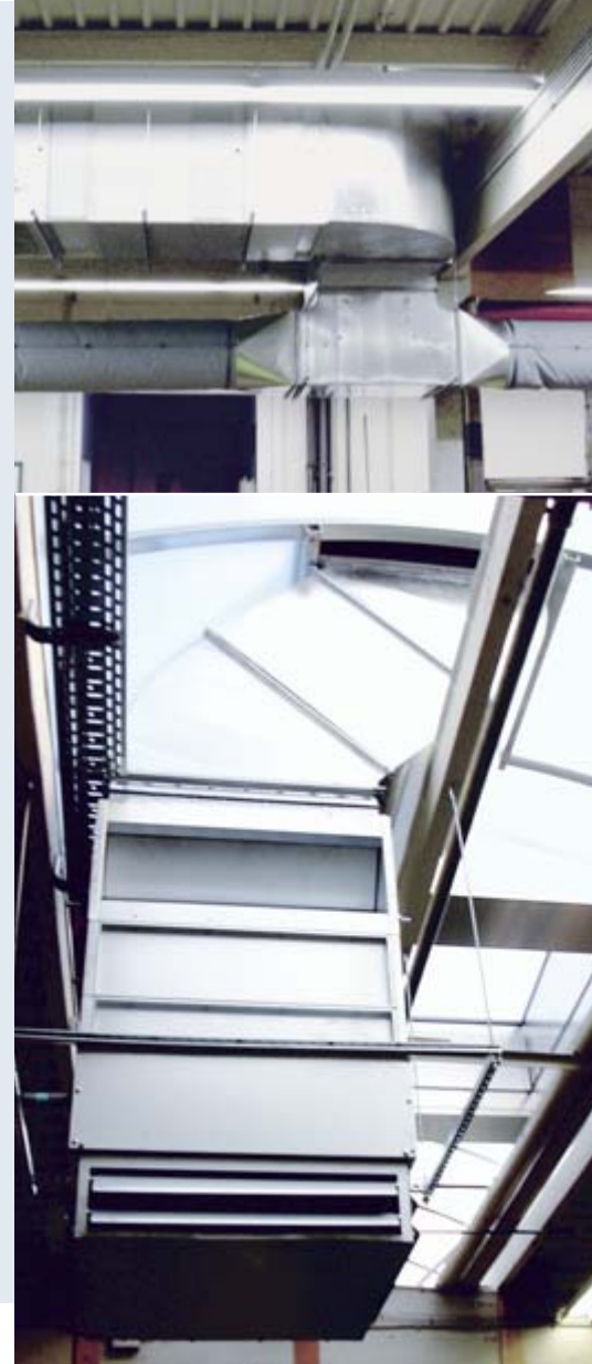
Air intake ducts for the internal fresh air units with integrated pumped warm water heating coils
