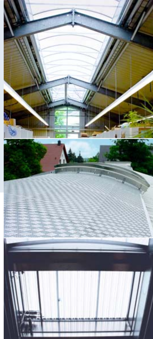
Perfect aeration and ventilation and best possible use of natural daylight (top)
