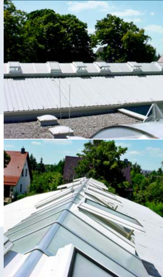
The old arcade rooflight caused dazzling effects and provided insufficient aeration and ventilation.
